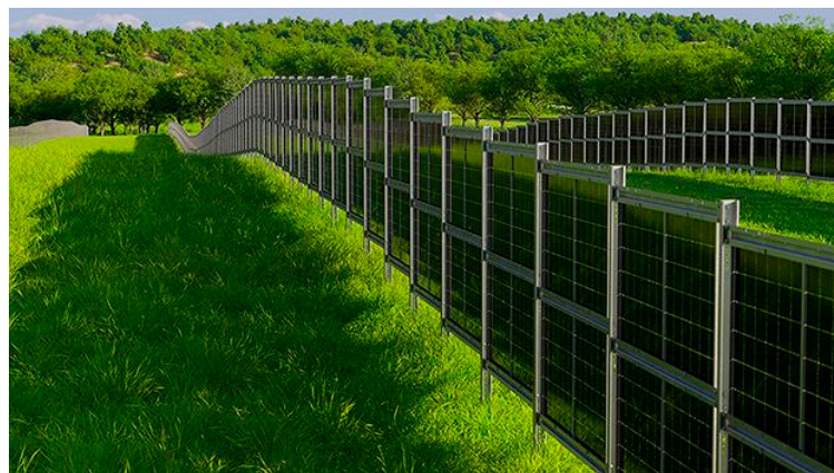
Figure 8. View of an APV installation using vertically mounted PV modules [53].
