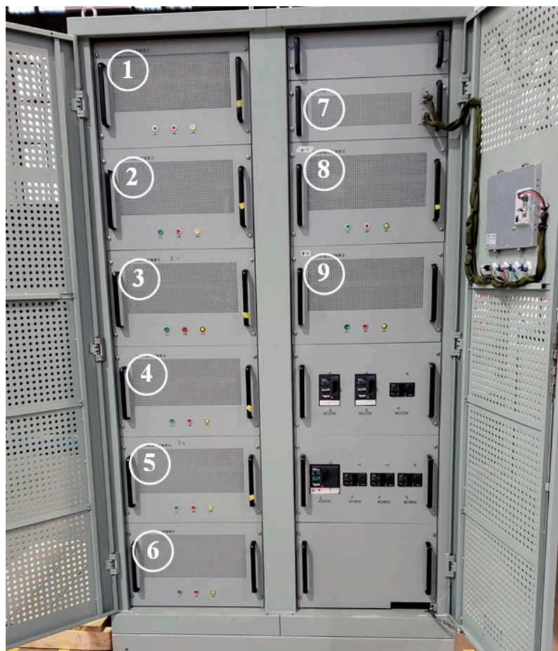
Figure A1. Seven-port router power cabinet based on DC bus.
