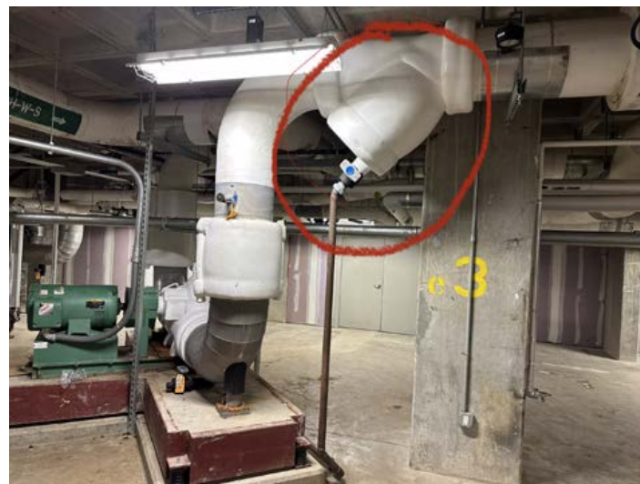
Figure 5. Zachry pump and strainer.
