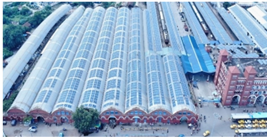
Figure 6. A 3 MW rooftop solar plant at Howrah Railway Station [50].
