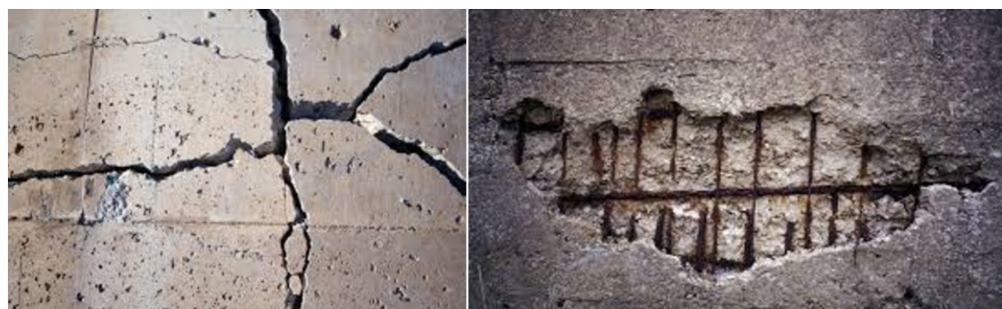
Figure 5. Fissuring and chipping due to element breakage in a marine environment structure (source: own collection).
