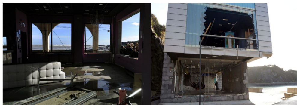
Figure 2. Buildings progressively damaged by extreme events. November 2010 storm (source: own collection).
