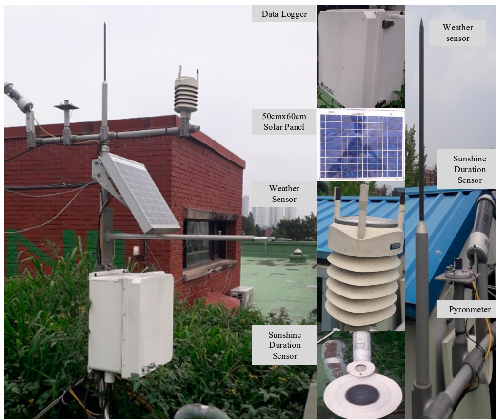
Figure 2. Various components of the weather station is shown in the pictures.
