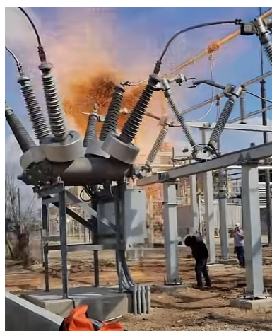
Figure 1. GIS spring circuit breaker explosion accident.
