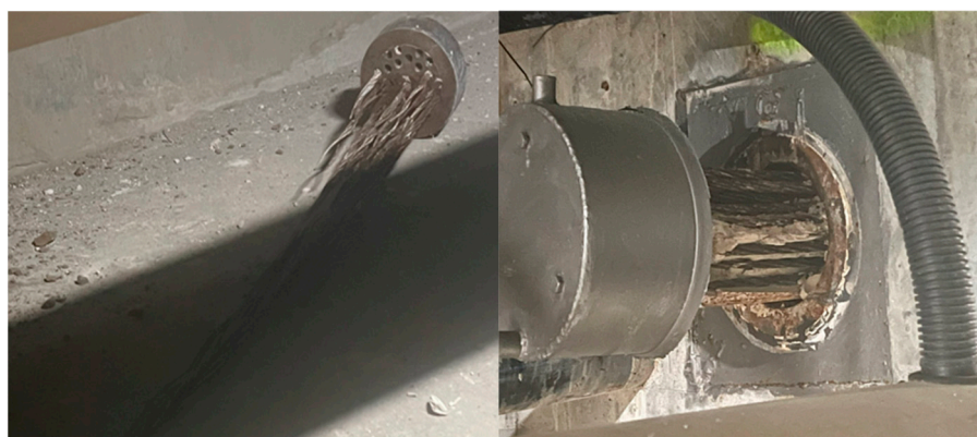
Figure 3. Documentation of breakup prestressing strand failure induced by localized steel corrosion inside the internal anchorage block (historical operational baseline: 2021–2024).
