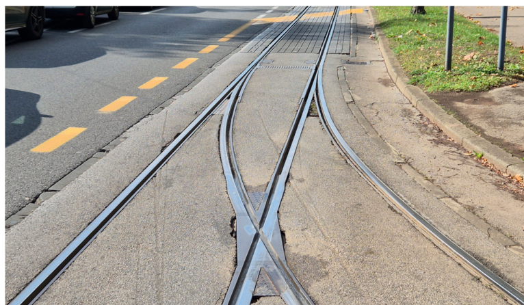
Figure 10. On-site photograph of the track defect corresponding to the consistently detected anomaly in Case Study 2.
