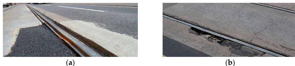
Figure 3. Illustrative examples of railway track defects: (a) degradation of road surface; (b) significant structural defect.
