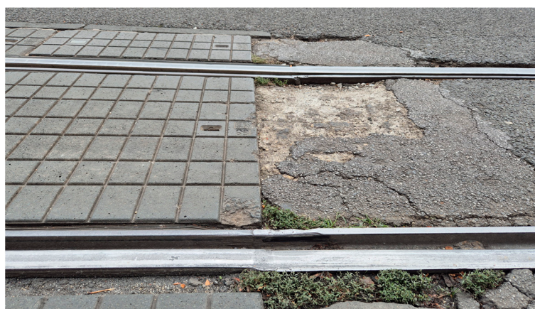
Figure 17. On-site photograph of the track defect corresponding to the consistently detected anomaly in Case Study 3.
