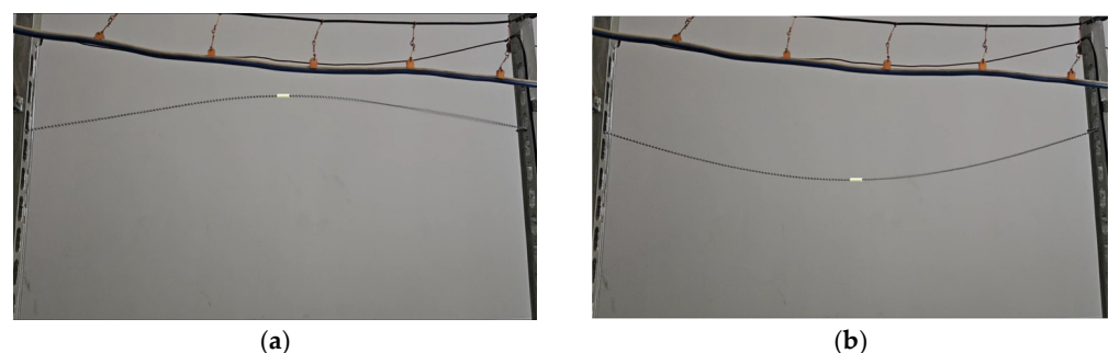
Figure 22. Frame of additional conductor galloping. (a) Highest point of additional conductor; (b) Lowest point of additional conductor.
