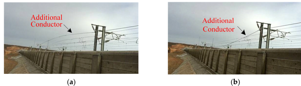
Figure 1. Additional conductor galloping of the Lanzhou–Xinjiang high-speed railway OCS in Baili wind zone. (a) Maximum galloping point; (b) Minimum galloping point.
