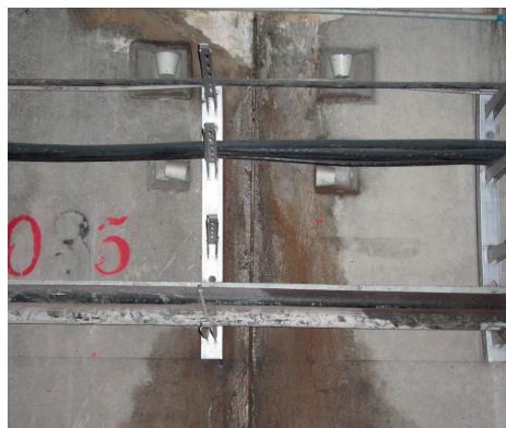
Figure 8. Water leakage image of the underground tunnel lining.
