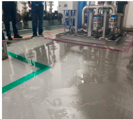
Figure 7. Water leakage image of the underground equipment room.
