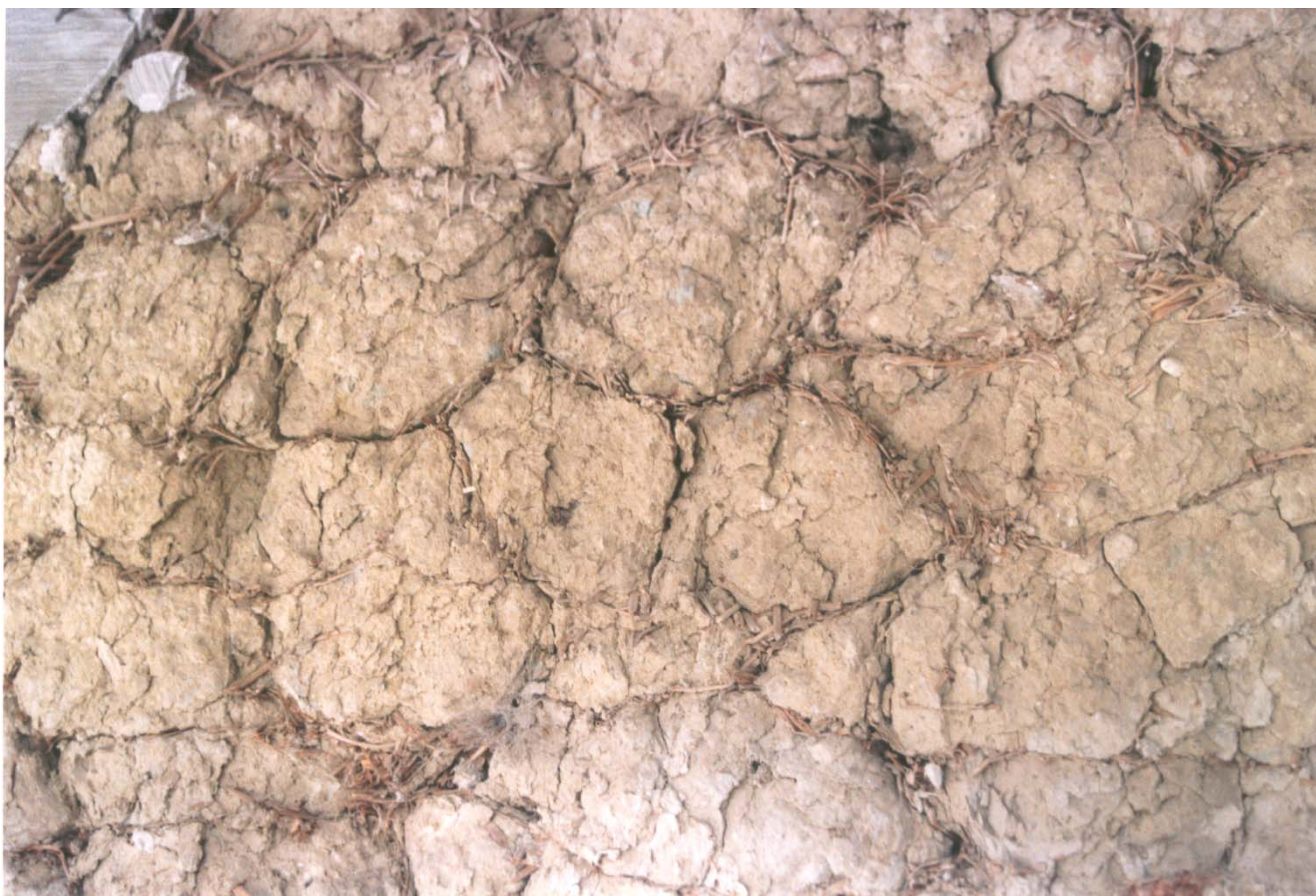
Figure 4. An external wall reveals the presence of cob bricks covered by straw.
