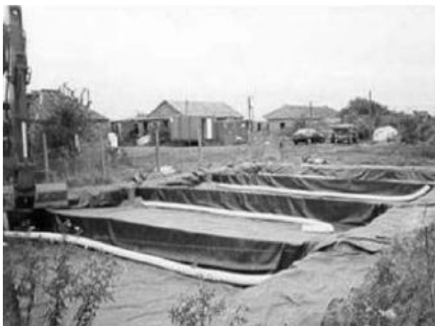
Figure 9. Construction of four pilot-scale cells in the site. Cell 1: untreated soil; Cell 2: EnvirOceM soil; Cell 3: OPC soil; Cell 4: ACT soil (from Jiangying et al. [38] with permission of Elsevier).
