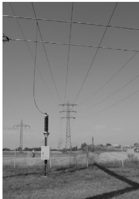
Figure 8. Signal coupling of the low-voltage signal to the high-voltage power line using a capacity post of the TFH equipment.
